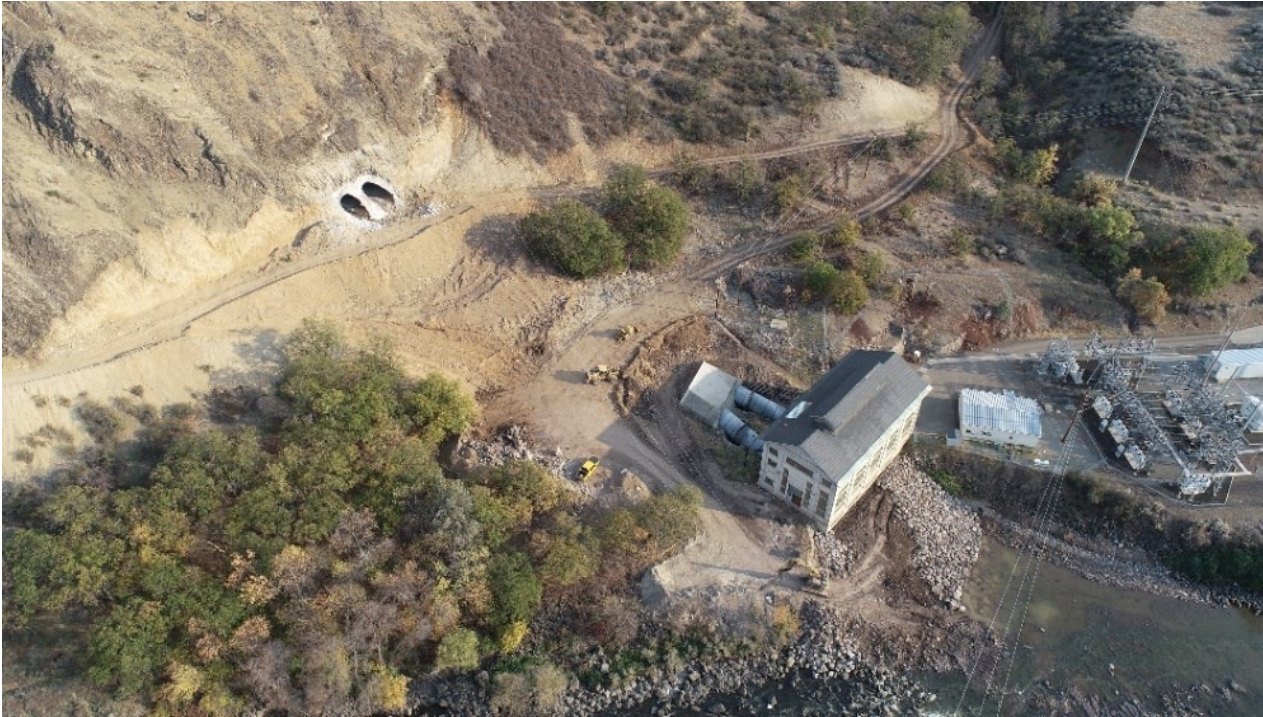
Copco 2 steel penstock thrust blocks have been removed. Lower thrust block backfilled. 1 November 2023
