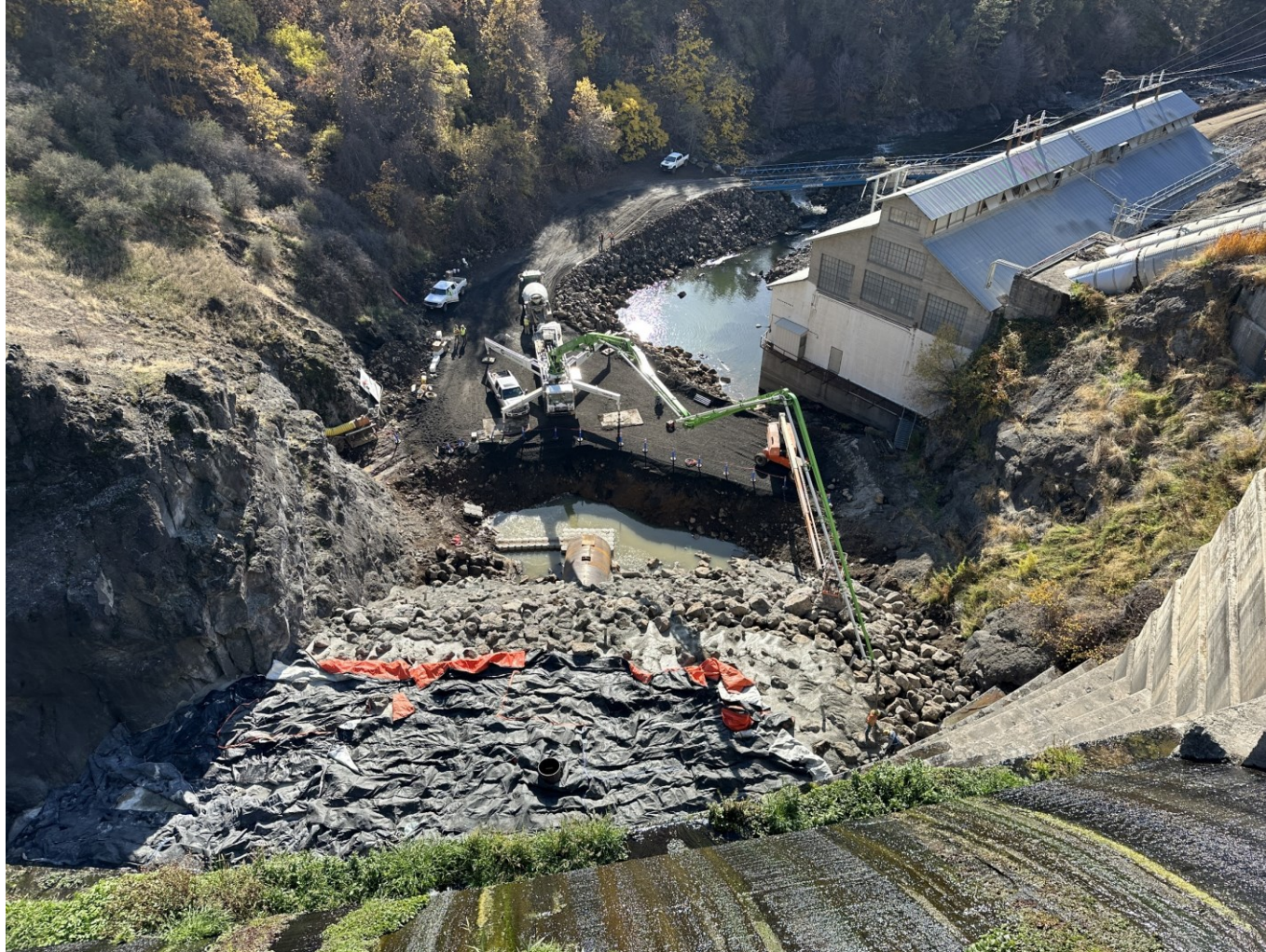
General view of Copco 1 dam and powerhouse with progress on grouted riprap placement over the steel extension pipe. 8 November 2023
